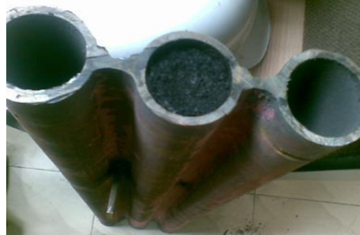
Figure 2 Blocked header tube
