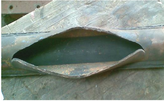
Figure 1 Ruptured boiler tube
